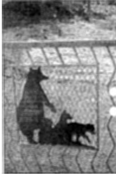
Wildlife railings lend interest to the bridge work over the new arroyo at Tramway Lane.
