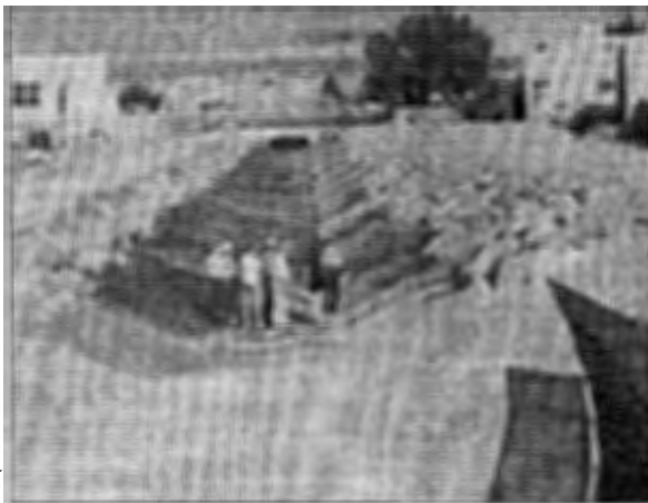
The North Domingo Baca Arroyo project is being completed between Tramway Lane and Boulevard just south of the Cedar Canyon subdivision by AMAFCA.
