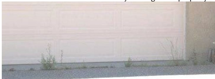
Don't let weeds occupy driveway cracks, giving your home an abandoned appearance and perhaps inviting suspicious activity.
