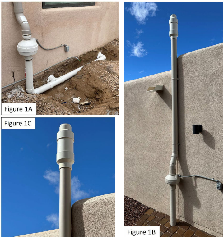
Figure 1: A trench for a “dual” approach (1A), the entire visible stack (1B) and close-up of exhaust vent muffler (1C).
